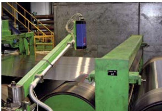
Abb. 8: Installation ASCOSpeed Reckanlage einlaufseitig ... Fig. 8: ASCOSpeed installation on the run-in side of the levelling unit ...
